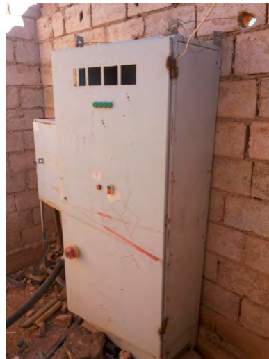
Figure 4. control panel is for a well located in the Azraq Basin area and under operation on a critical point of lack of water supplied to consumers
