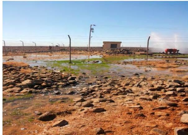
Figure 3. Water loss due to pipe leakage leaking water for long time in Pic
