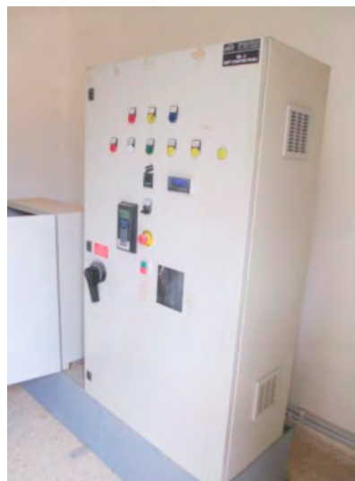
Figure 5. 15 years old well control panel in Disi-Aqaba area under an operation of a private company
